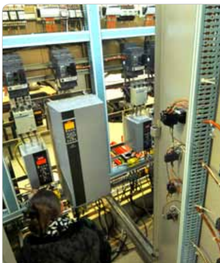
Electrical cabinet - Automatic control and supervision of the facilities
